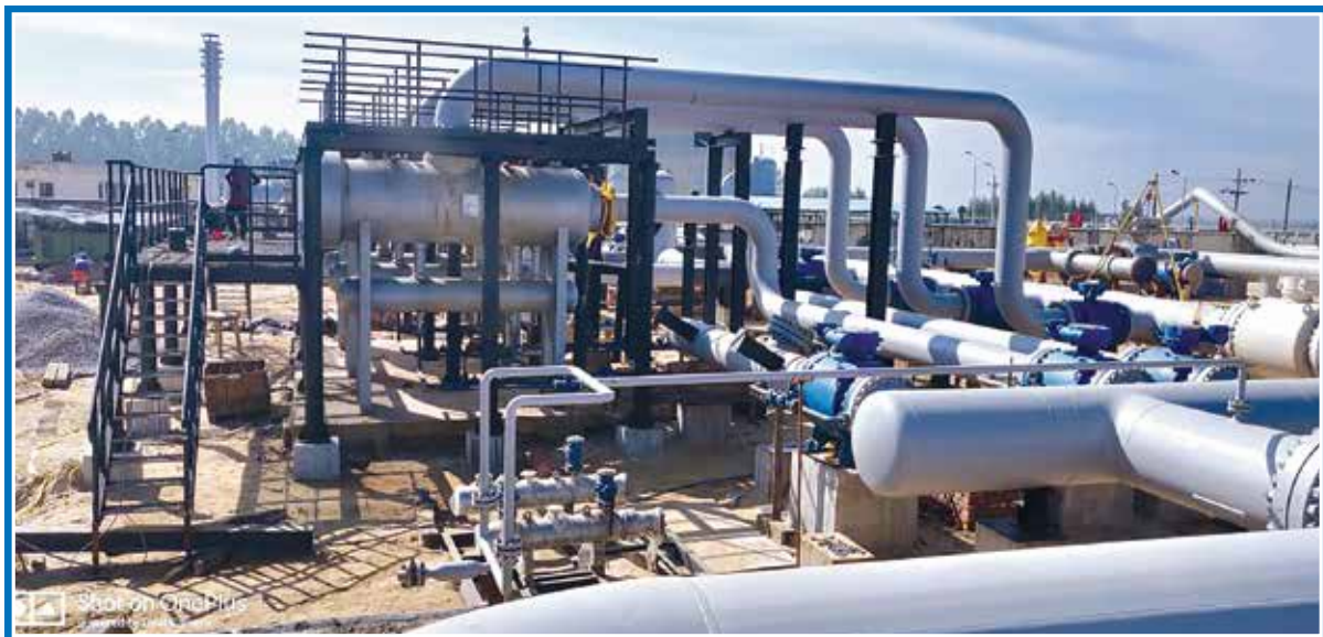
1500 million cubic feet capacity metering station constructing under Maheshkhali Zero point project
