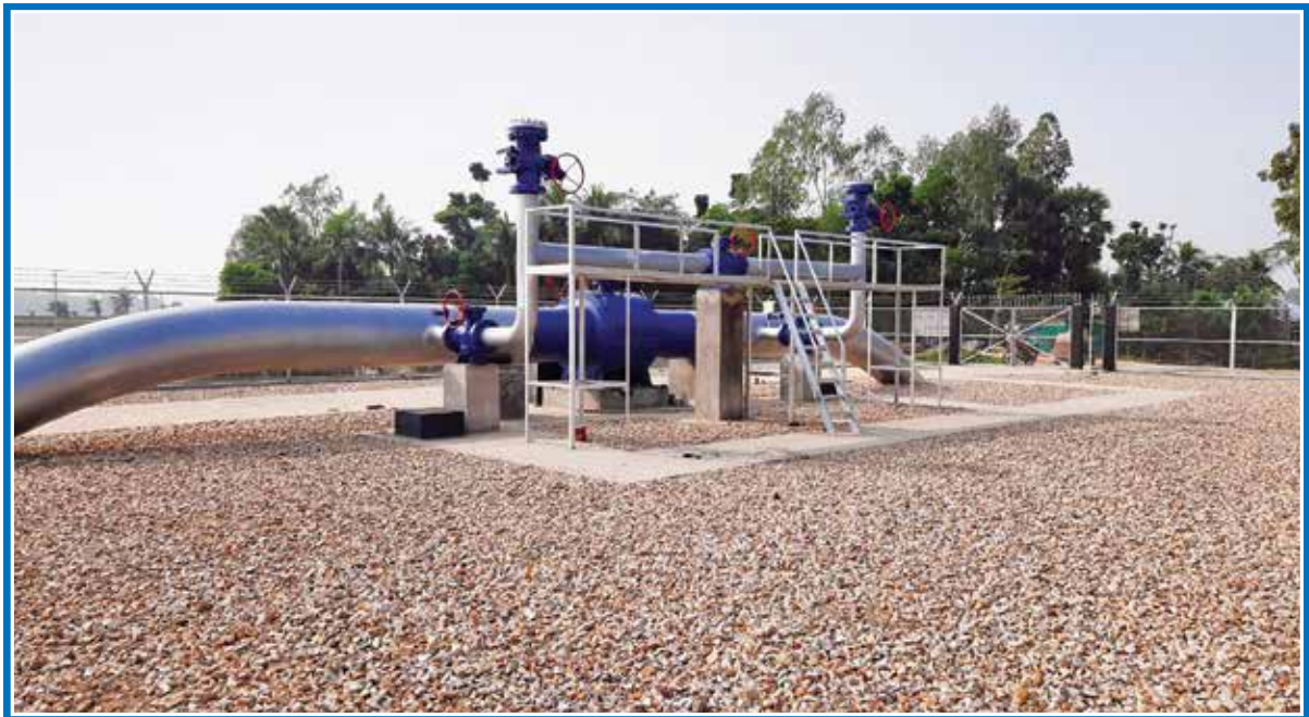
Valve Station Under Chattogram-Feni-Bakhrabad project
